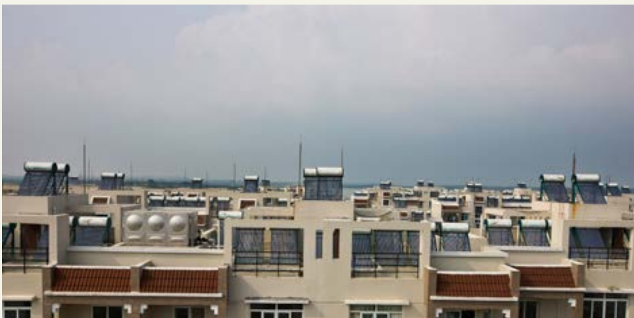
Solar panels, Wuhan City, China
